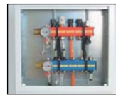
Heating circuit distributor
