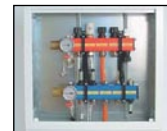
Heating circuit distributor
